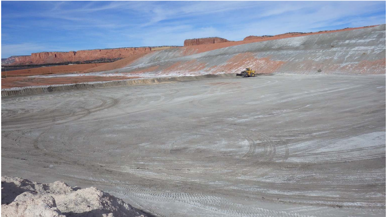
Photograph 1: Typical Deposition Area Condition
