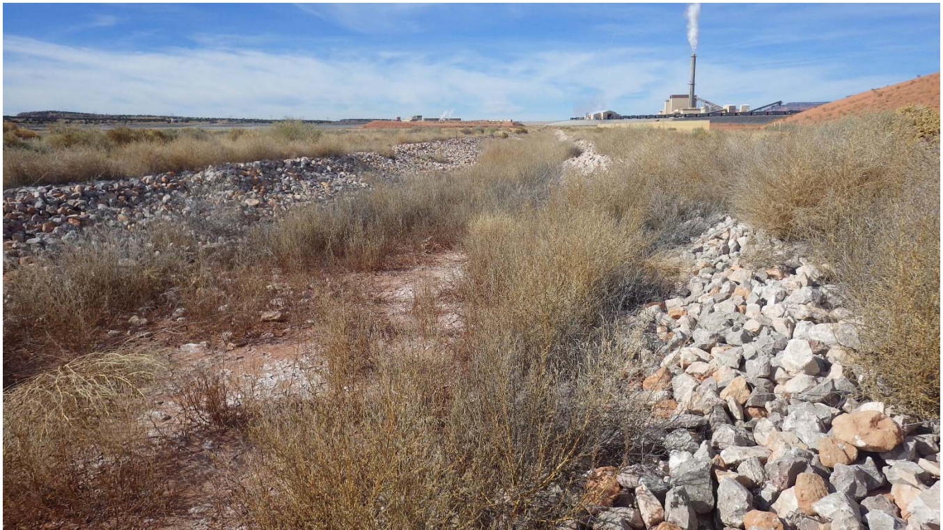
Photograph 5: Typical Storm Water Channel Condition
