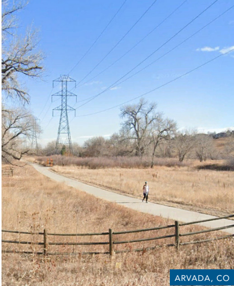
Facility: Tap-Ridge and Lookout-Ridge 230kV Transmission Line
