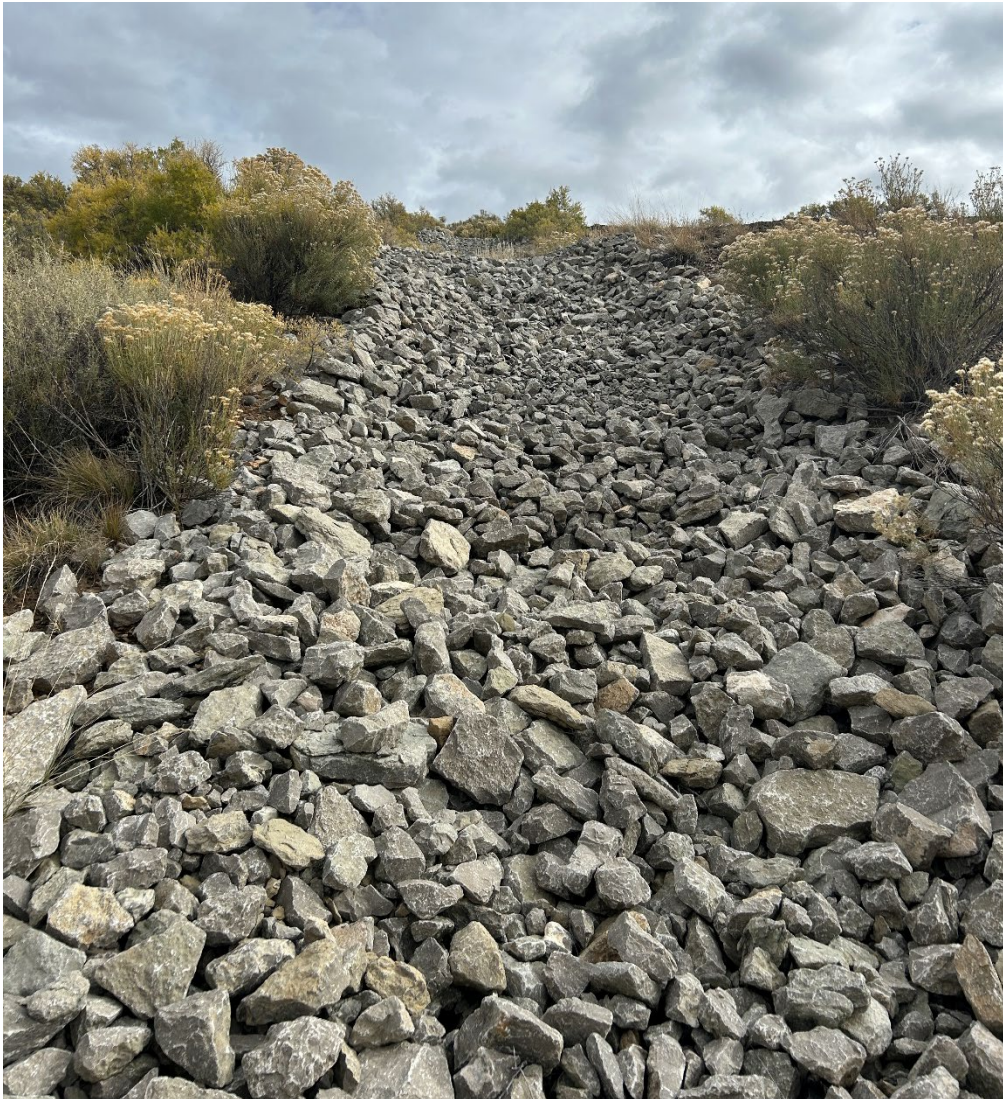
Photograph 6: Typical Condition of Downchute Channels
