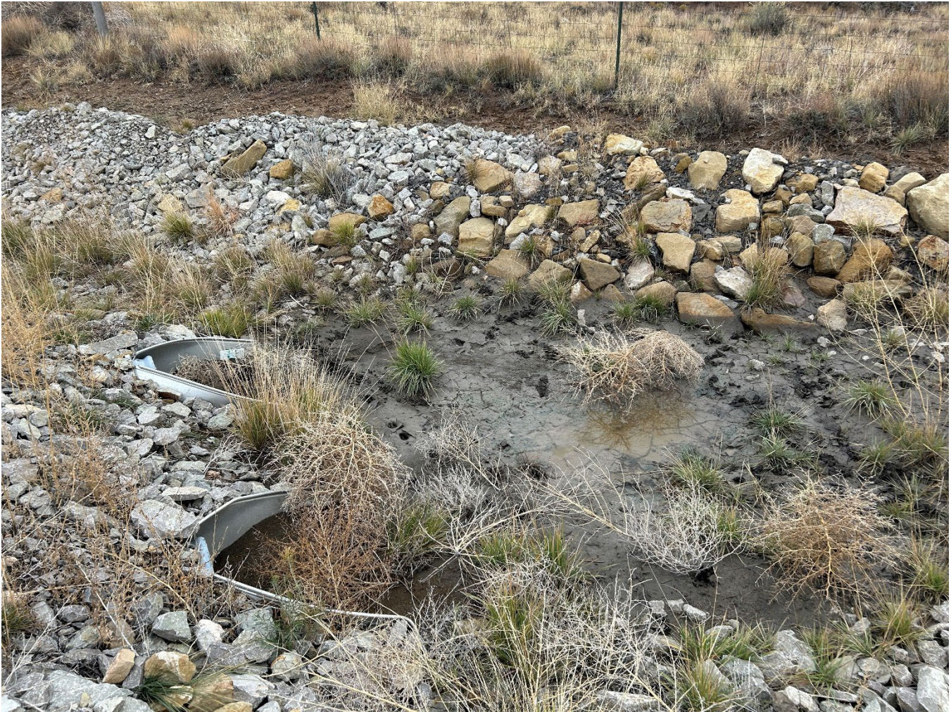
Photograph 11: Sediment Buildup at Downstream End of Culverts
