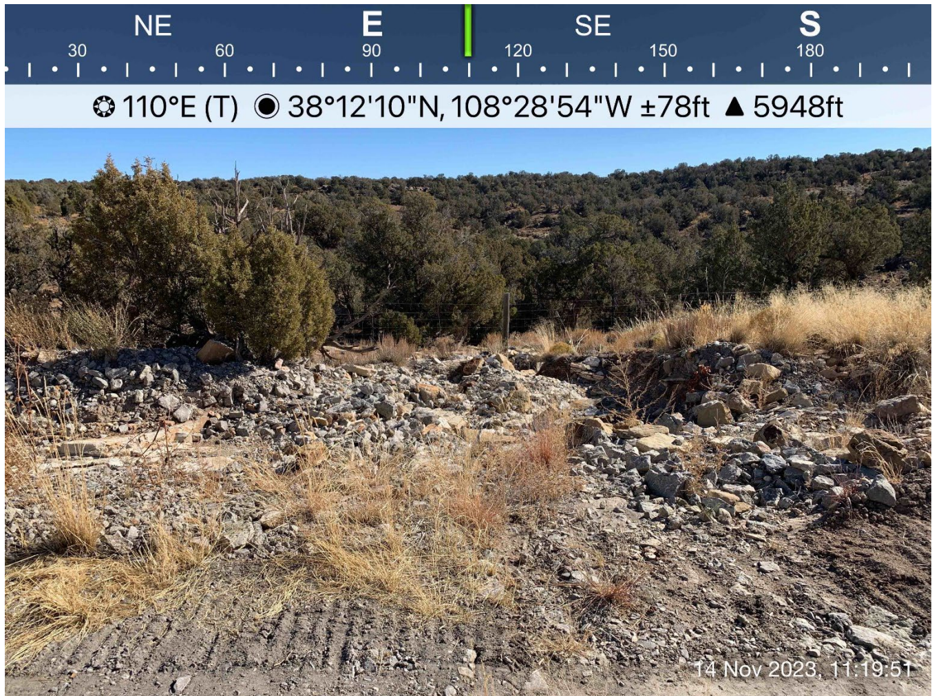
Photograph 9: Damage to Stormwater Outfall
