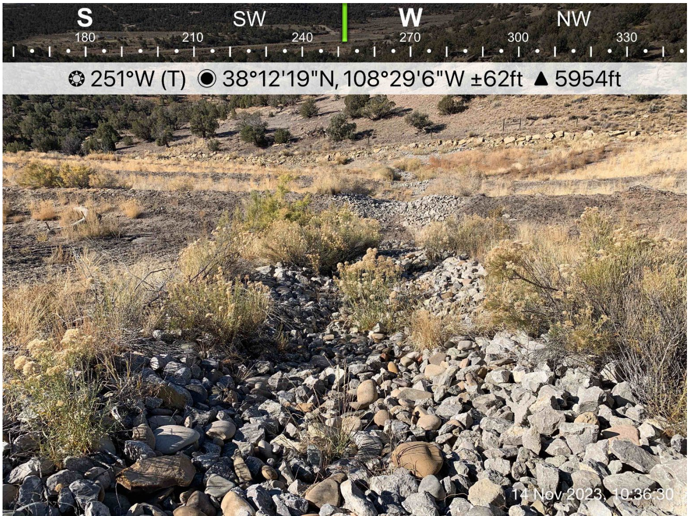
Photograph 6: Typical Condition of Downchute Channels
