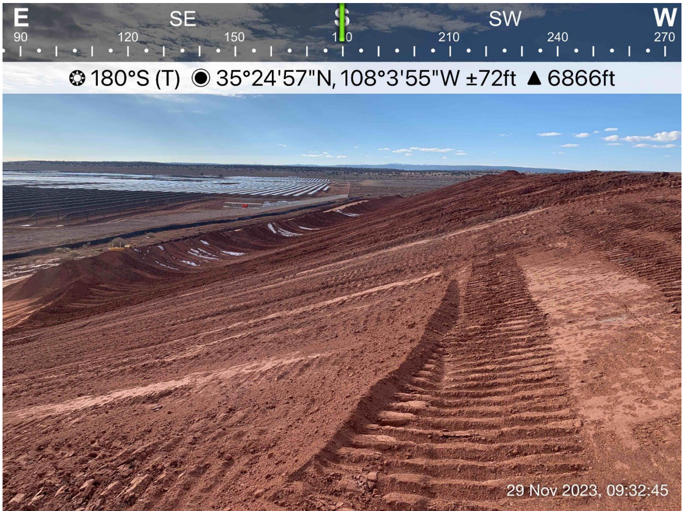
Photograph 4: Condition of the East Embankment Slope at the Time of the Visual Observation
