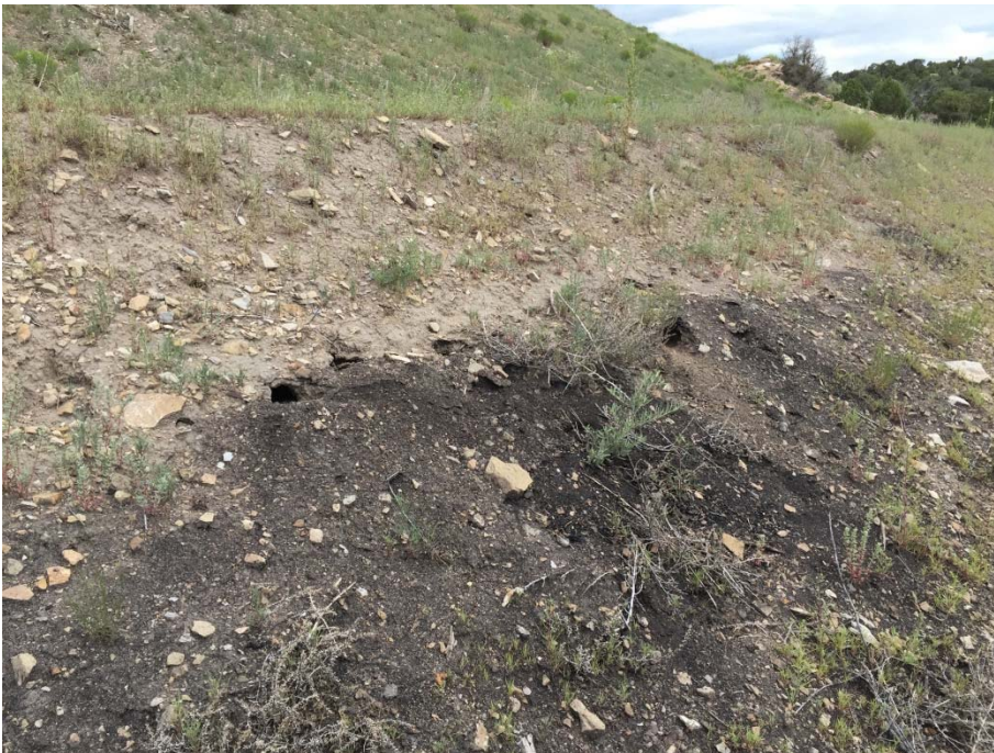
Figure 4: Animal Burrows on Embankment Slope
