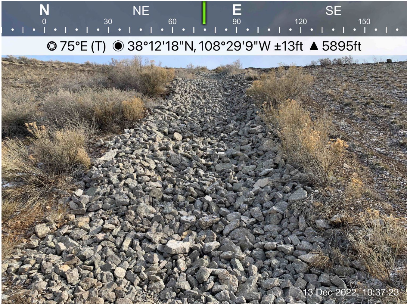
Photograph 7: Typical Condition of Downchute Channels
