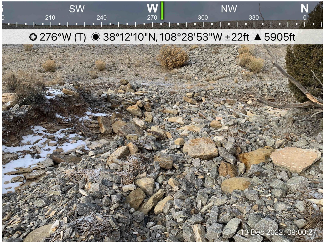
Photograph 10: Damage to Stormwater Outfall
