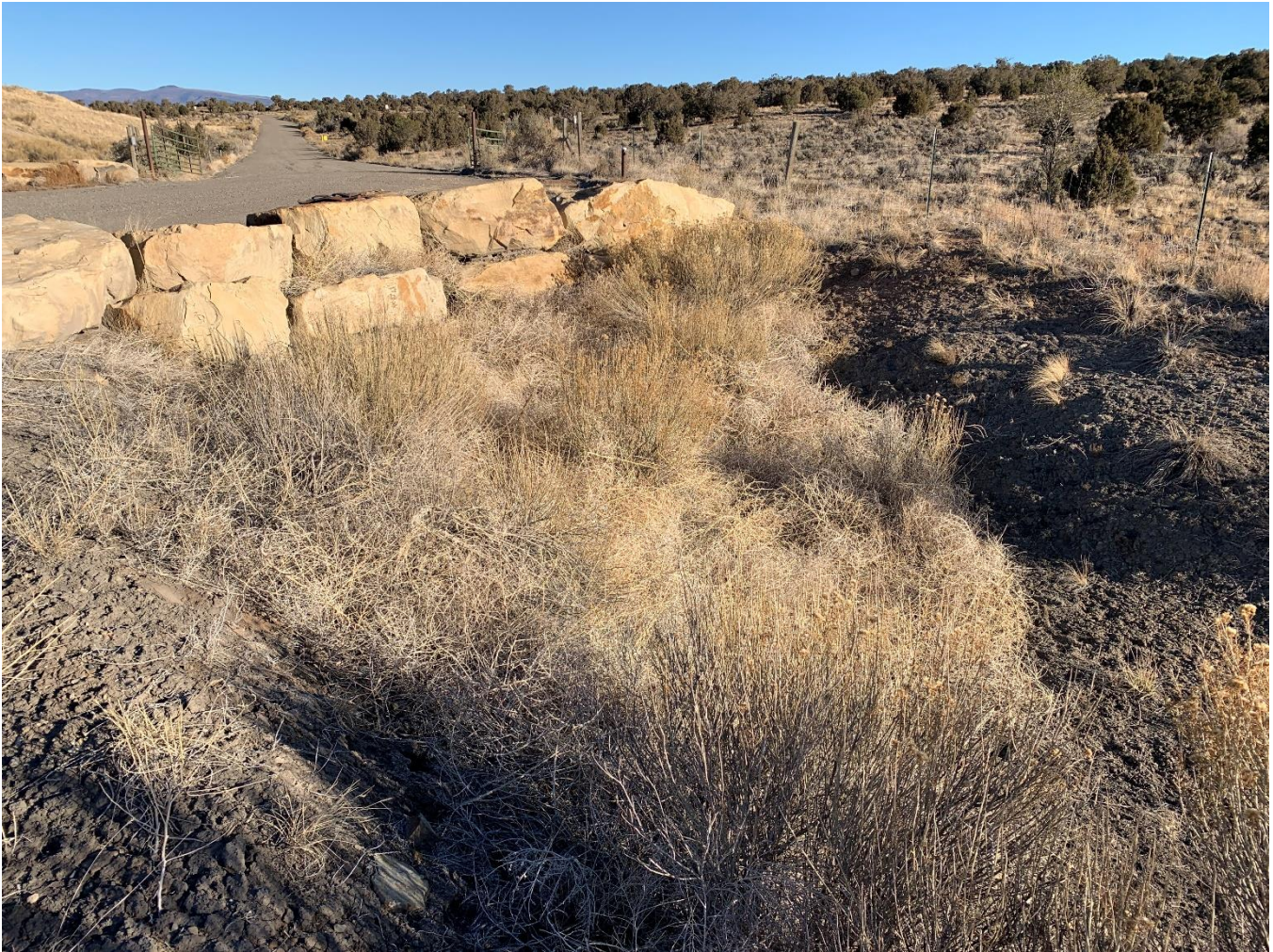
Photograph 8: Buildup in the East Perimeter Channel at the Downstream Ends of the Culverts
