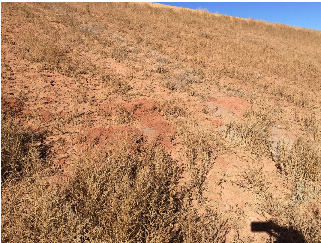
Photograph 5: Animal Burrows on East Embankment Slope
