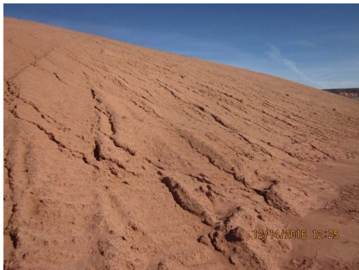
Figure 5: Minor Erosion Rills on South-embankment Slope
