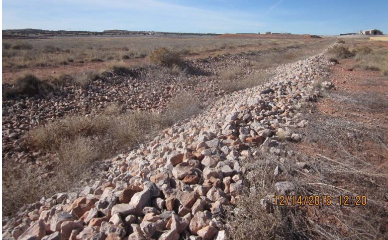
Figure 7: Typical Storm Water Channel Condition
