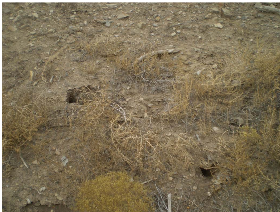
Photograph 4: Animal Burrows on Embankment Slope
