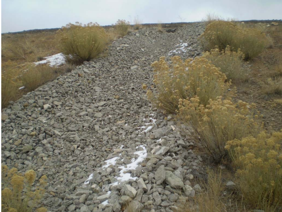
Photograph 6: Typical Downchute Channel Condition
